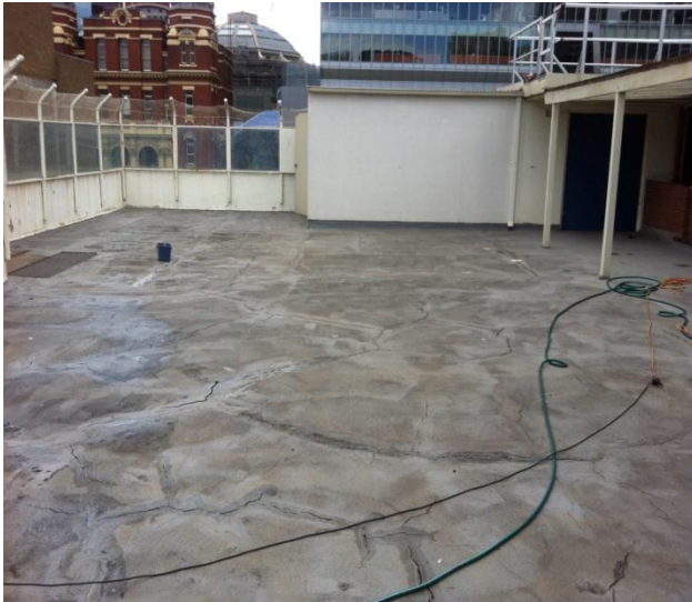
Original cracked & leaking roof membrane
