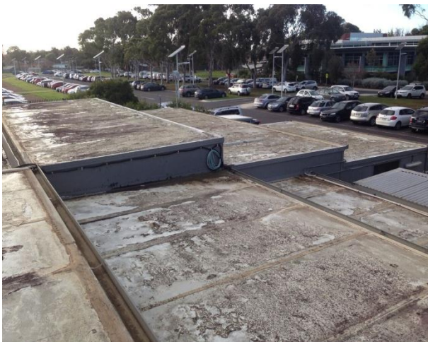
Original leaking roof membrane
