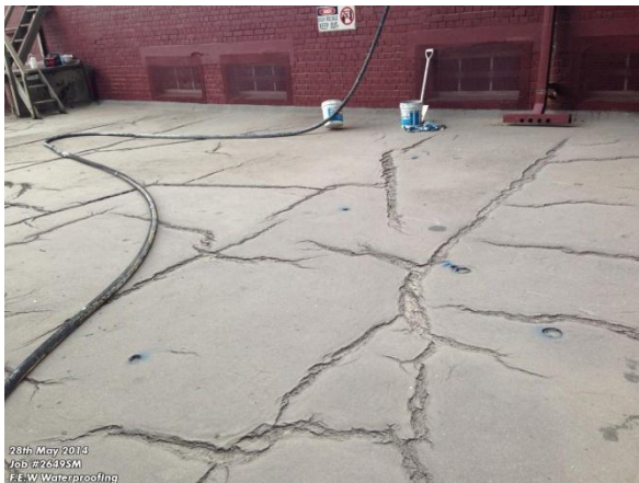
Original cracked & leaking roof membrane
